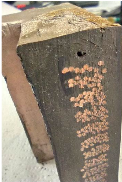
Failed Dry-type MV winding
